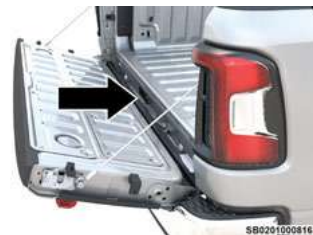
Wiring Access Hole
