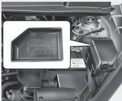
Engine compartment fuse panel
