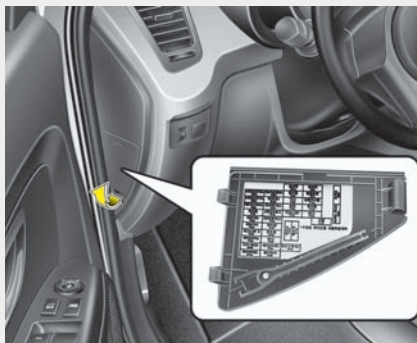
Inner fuse panel
