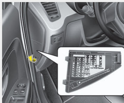
Inner fuse panel
