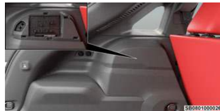
Rear Power Distribution Center Location
