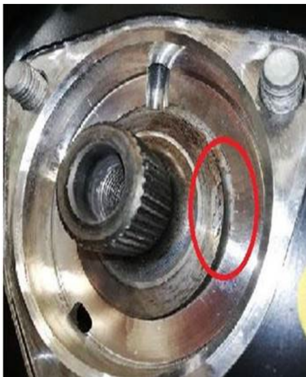
Figure 4: Metallic particles/damage in the wheel hub/bearing.
