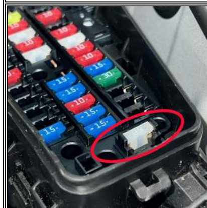
No Good (not secured)
