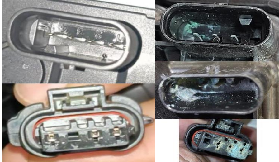
Fig 1. Normal condition left. Corrosion on right.
