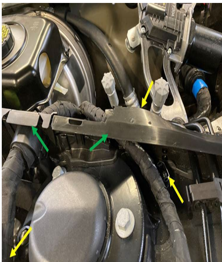
Figure 1: Plenum chamber covers (green arrows).
