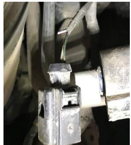
Figure 1. N280 control wire damaged at T3r connection
