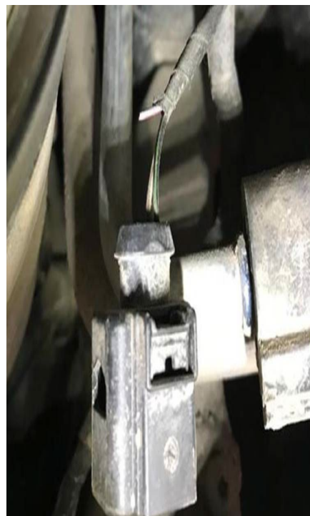
Figure 1. N280 control wire damaged at T3r connection
