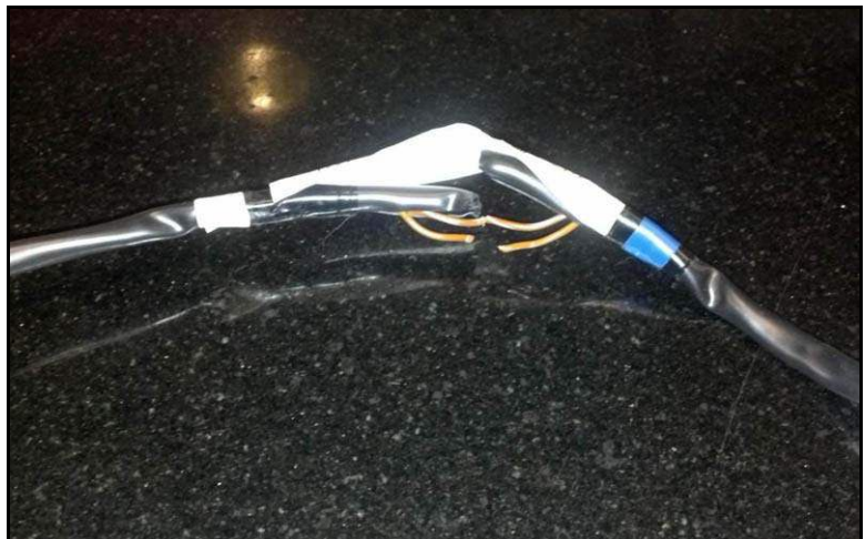
Close-up View of Damaged Harness
