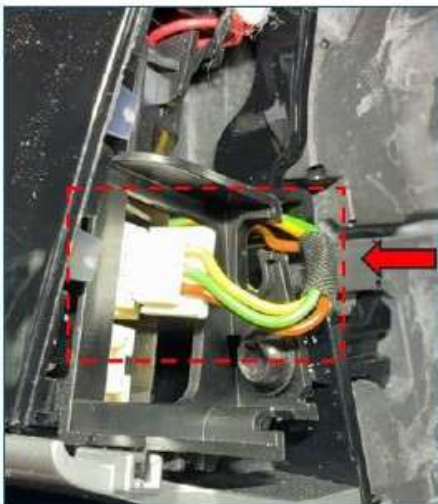
Figure 1. Incorrect wire routing.
