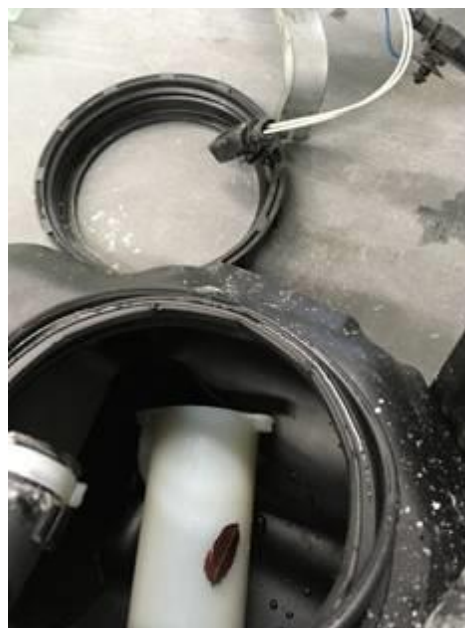
Figure 2. Filter element housing loose inside tank.
