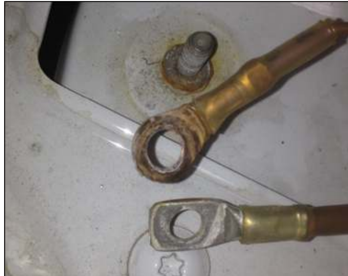
Figure 2 – Example of corrosion on ground point
