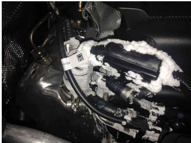
Figure 1. Evidence of leak—AdBlue residue.
