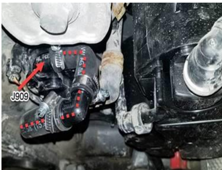
Figure 9. Closer look at the connections.
