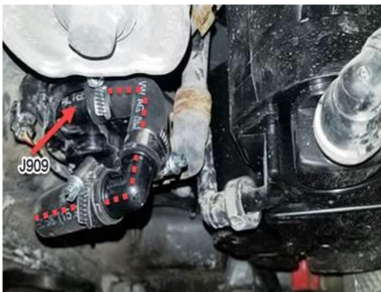
Figure 9. Closer look at the connections.
