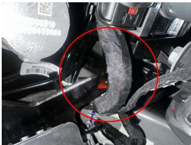
Fig. 1 Incorrectly Routed Harness
