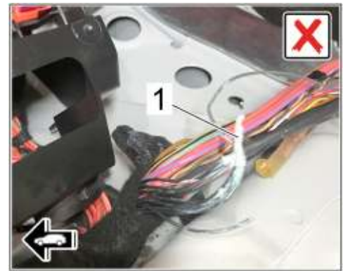
Corroded splice connection (shown as an example)
