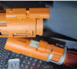
Improperly connected HV connectors
