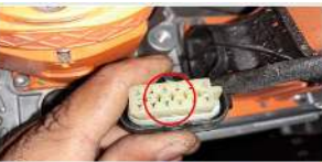
Corrosion on interlock pins on HV component's low voltage connector
