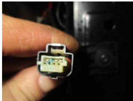
Figure 5: Oxidation on the connector housing.
