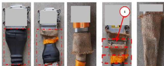
Fig. 3 HV Cable Harness Exposed Metal Mesh Shielding
